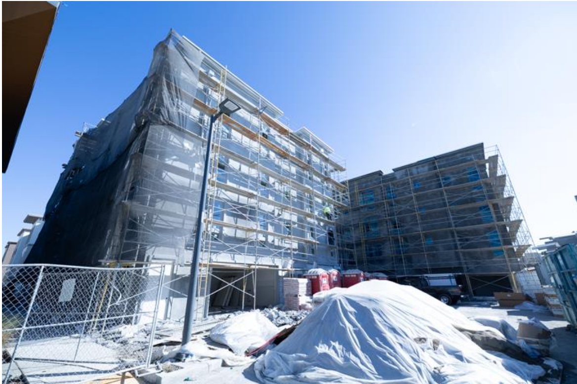
Figure 6: A 5-storey multi-residential building under construction utilising a prefabricated stud framing solution.
