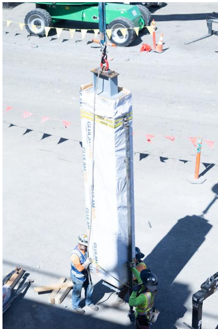
Figure 10: The Java offices utilised a proprietary steel connector to transfer vertical loads from column to column without crushing floor panels.
