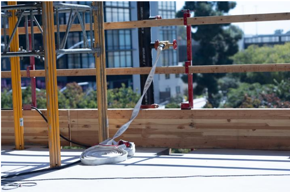
Figure 16: A temporary fire hydrant is installed in a mid-rise mass timber project, and will be removed once the building's permanent fire hydrant is installed and operational. While this hydrant isn't required by local authorities, the builder believes it is a simple risk mitigation strategy to avoid potential significant consequences of a loss event occurring.
