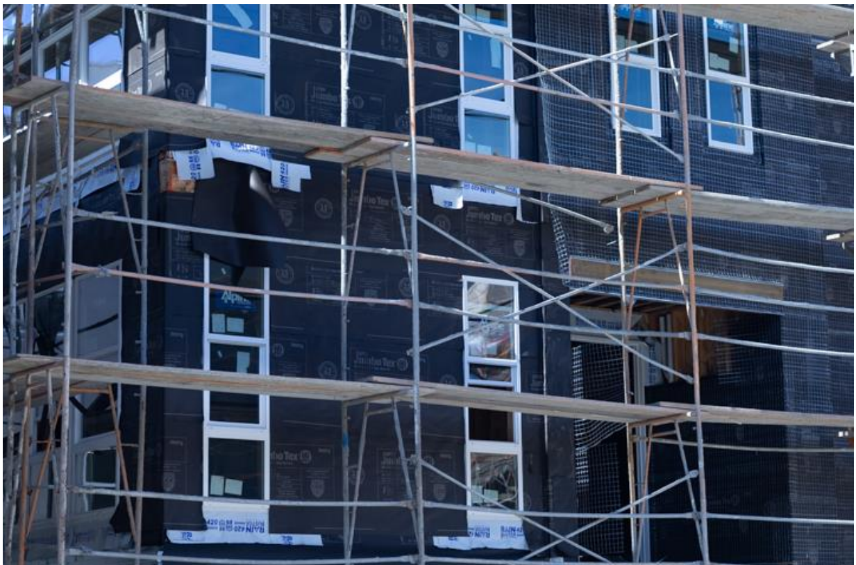
Figure 18: This 4 storey prefabricated timber frame apartment building utilised Super Jumbo Tex – a vapour permeable, water resistant membrane used in the building envelope.
