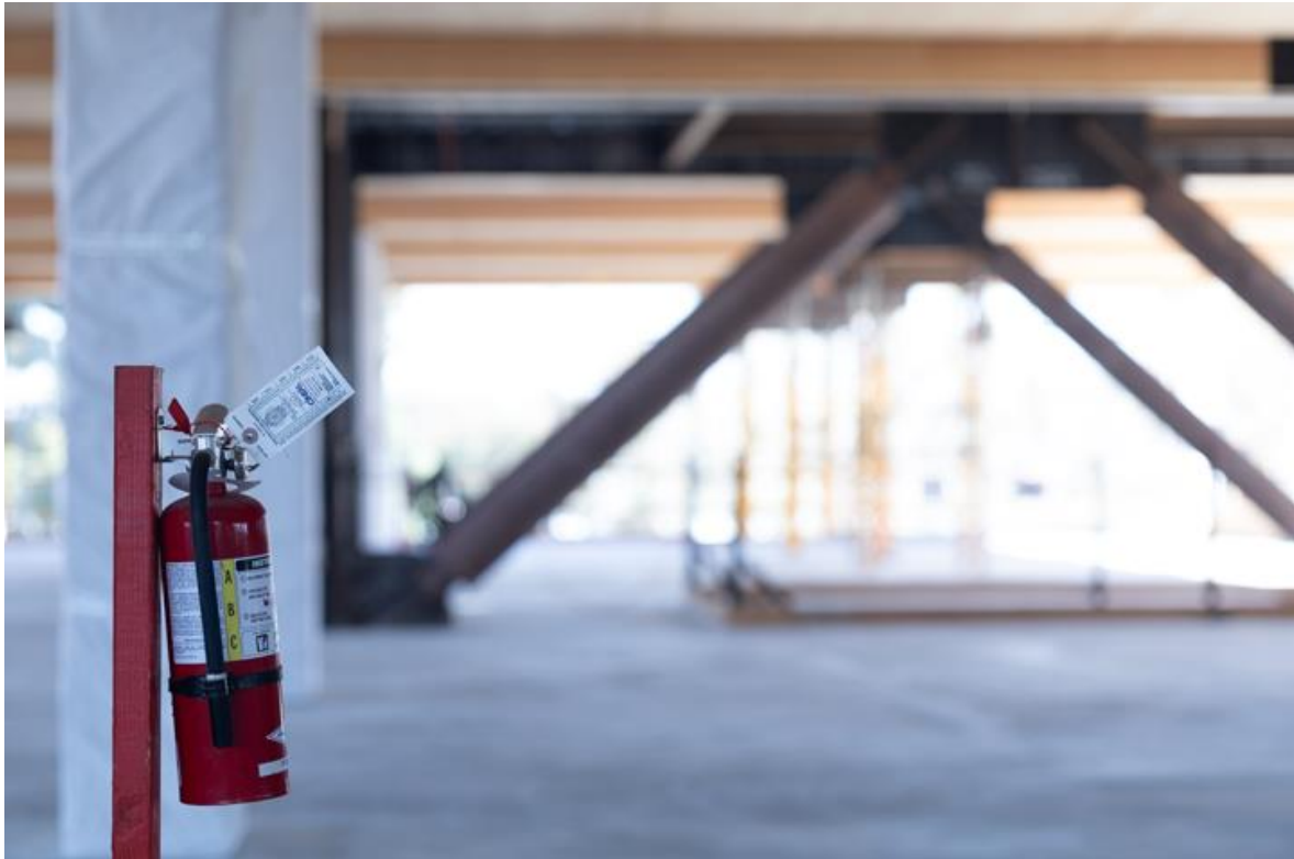
Figure 15: A fire extinguisher presents a simple, mobile form of fire safety. While useless against established fires, this might be used to address a small fire in its early stages.
