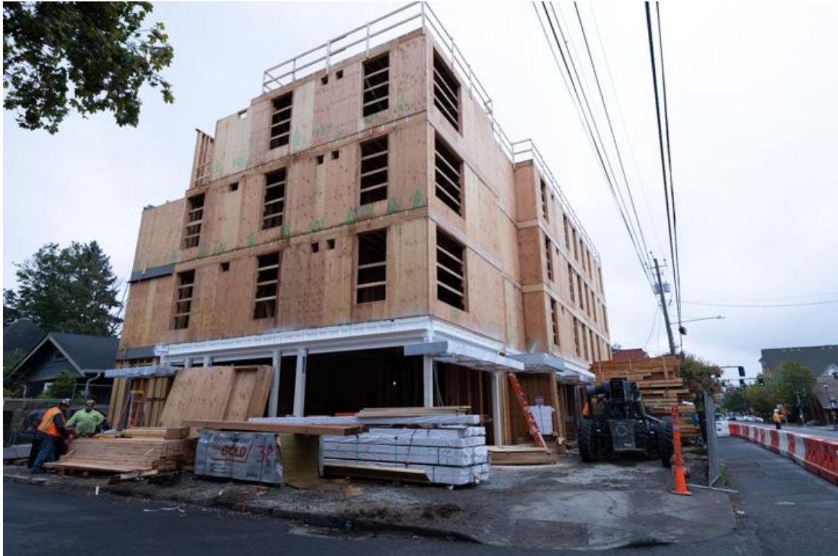
Figure 11: This four-storey apartment building in Portland Oregon effectively uses a structural steel frame to create large open spaces on the ground floor, with timber frame apartments above.
