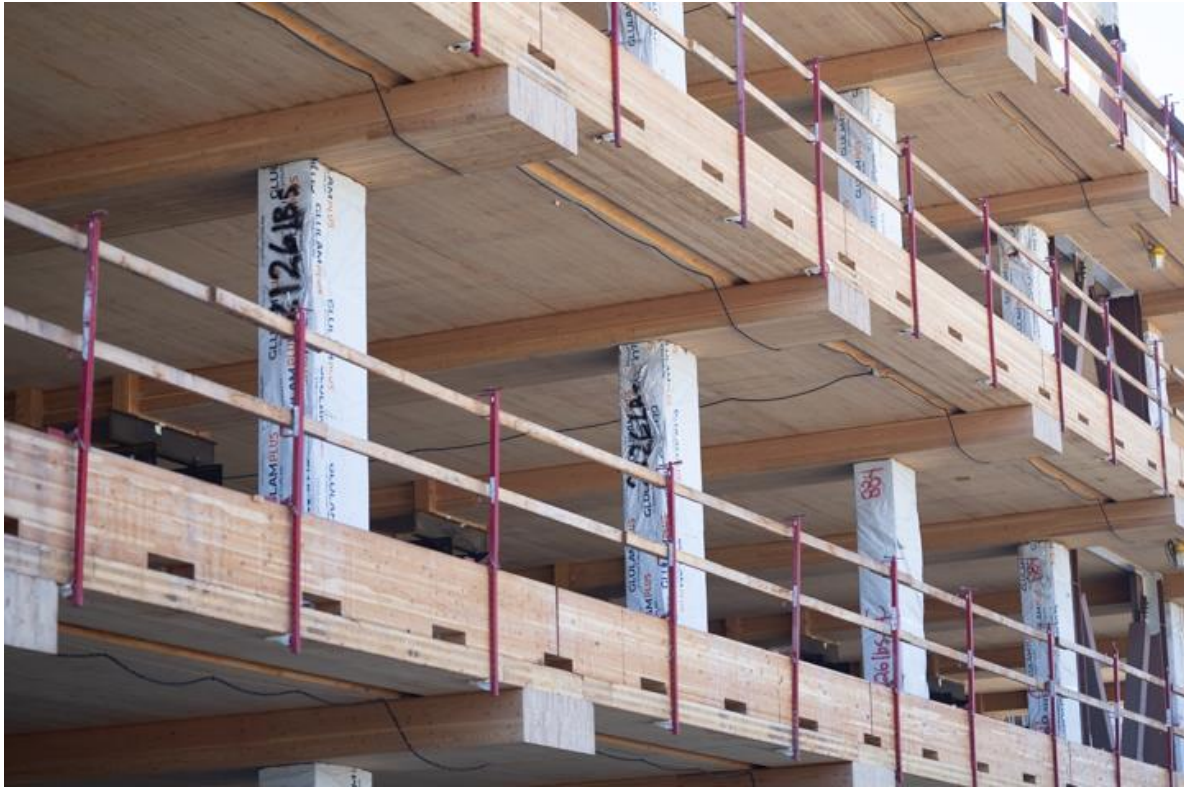
Figure 8: Vertical loads are directly transferred to the foundation by ‘stacking’ them from floor to floor, as shown in this mid-rise office project.
