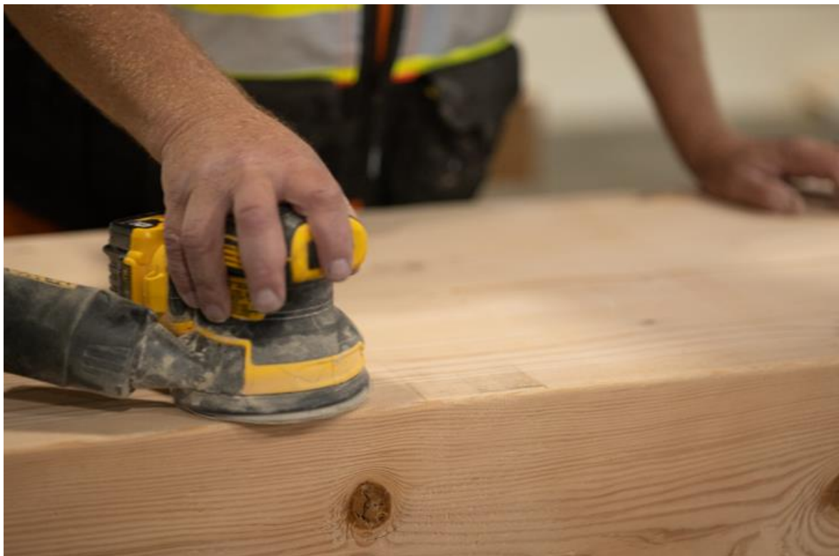
Figure 17: While this Glulam was being pre-sanded in the shop before leaving for installation, the supplier (Timberlab) advised that it would likely still need to be spot-sanded on site.
