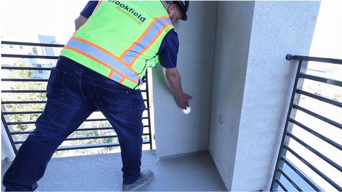
Figure 19: The Superintendent of this Brookfield Residential site points to the permanent vents installed in external wall build ups to ensure they are able to dry out in the event of moisture ingress.
