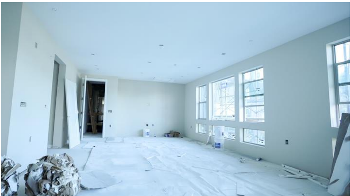
Figure 12: This 5 storey prefabricated lightweight framed apartment building utilised a pourable Gypcrete floor topping to counter airborne noise transfer.
